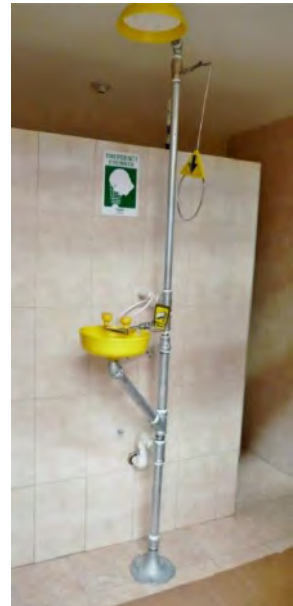
Emergency shower and eye wash station
