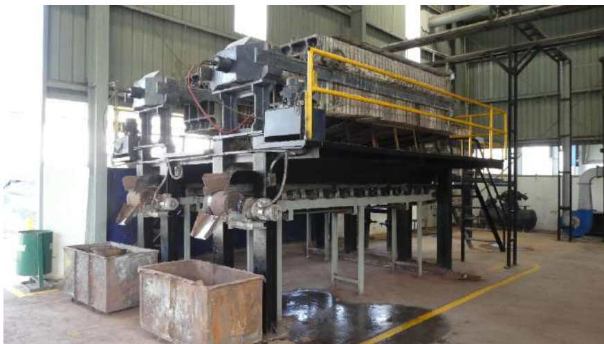
Filter press removes suspended particulates from the electrolyte
